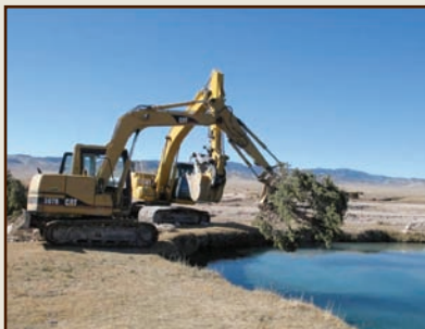
Local natural materials were used to restore and stabilize the spring source pool.
