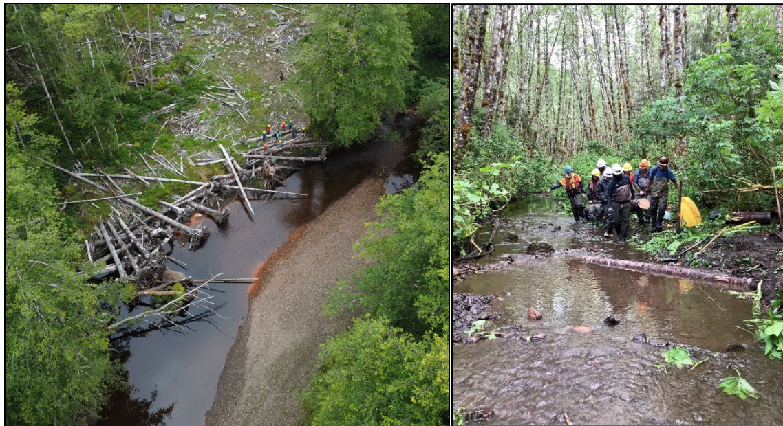
Figure 5: Crews in the Tongass National Forest used large woody debris to slow stream bank erosion (left) and stabilize the stream bed (right) in the Margaret and Ward creek watersheds to improve fish habitat.
